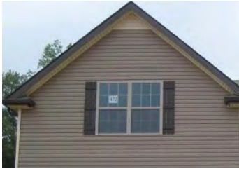
12” shutter flanking a 6’ window and there is no trim around the window – not allowed.
